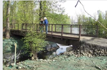
A new bridge was installed at Whitaker Ponds to improve water connectivity between the ponds and the Slough.
